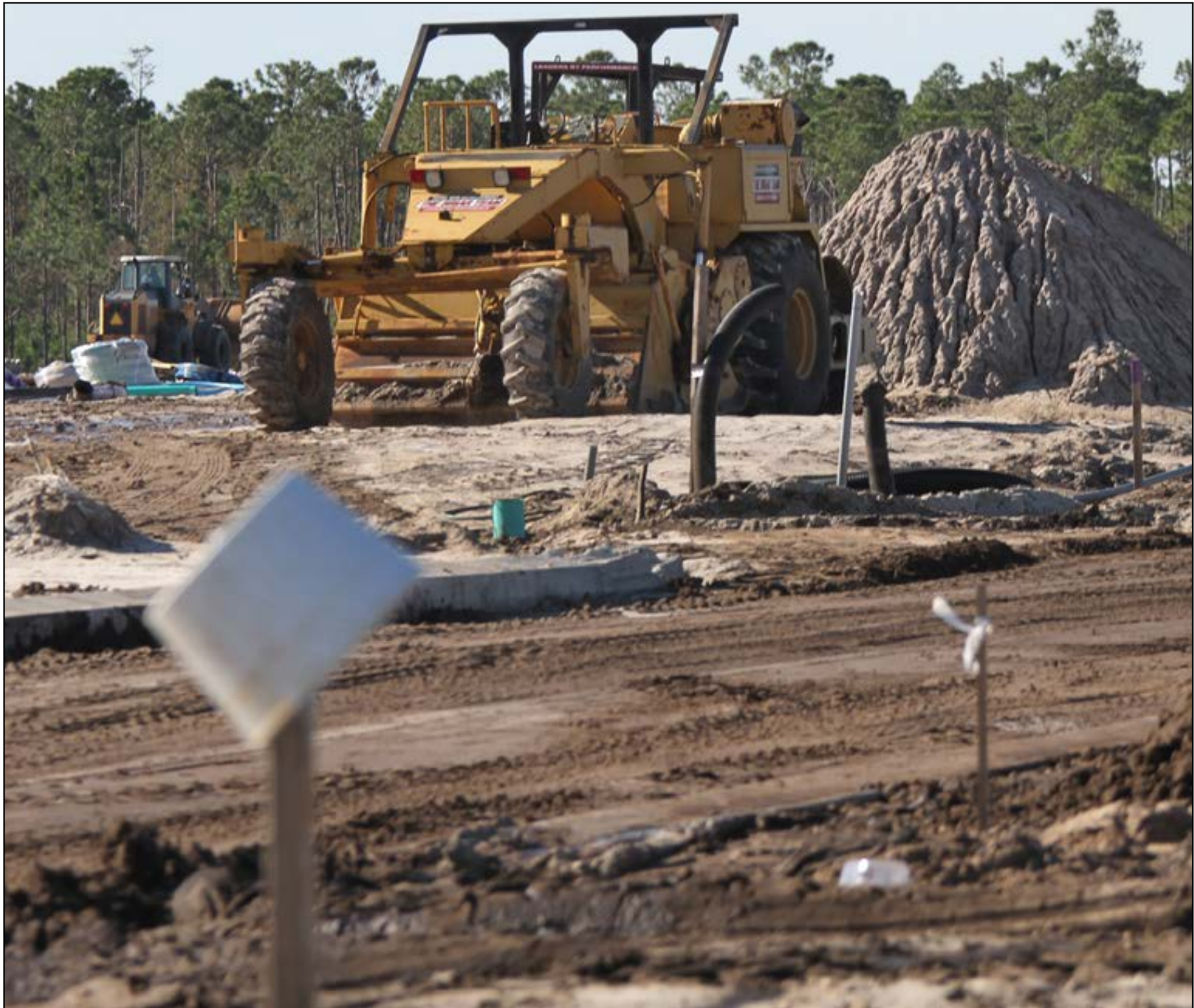
Infrastructure work proceeds on ICI Homes' planned 1,200-home Mosaic "full life community" west of LPGA Boulevard. ICI Homes recently agreed to pay $21 million to acquire 1,020 acres of timberland on the south side of Granada Boulevard/State Road 40, west of Tymber Creek Road, where they also plan to build a "full life community." [NEWS-JOURNAL/DAVID TUCKER]
